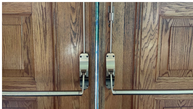
Figure 13: Missing Weatherstrip – Main Entrance Door
