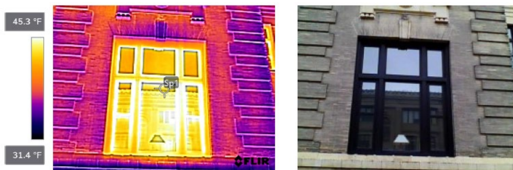
Figure 11: Infrared Image of Window on Northwest Wall of Building
