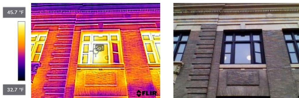
Figure 10: Infrared Image of Open Window Observed During Assessment
